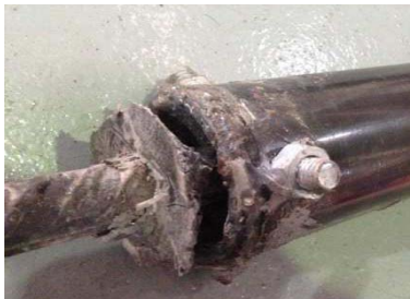
a) Grout-bar failure
